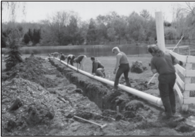
INTO THE TRENCH: Position one person at each joint before dropping the pipe in the trench.
